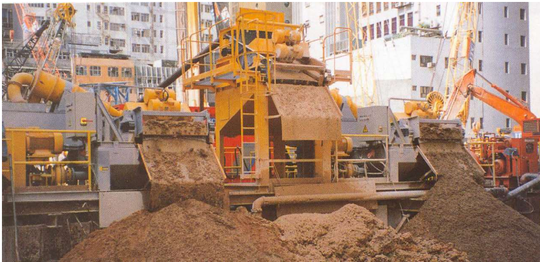
Figure 5-29 De-sanding plant for bentonite slurry
