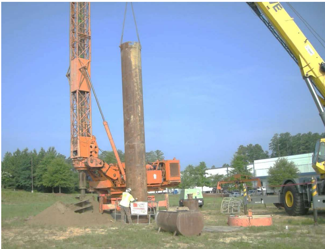
Figure 5-2 Inserting Casing into an Open Hole Prior to Rock Excavation at a Site in Georgia
