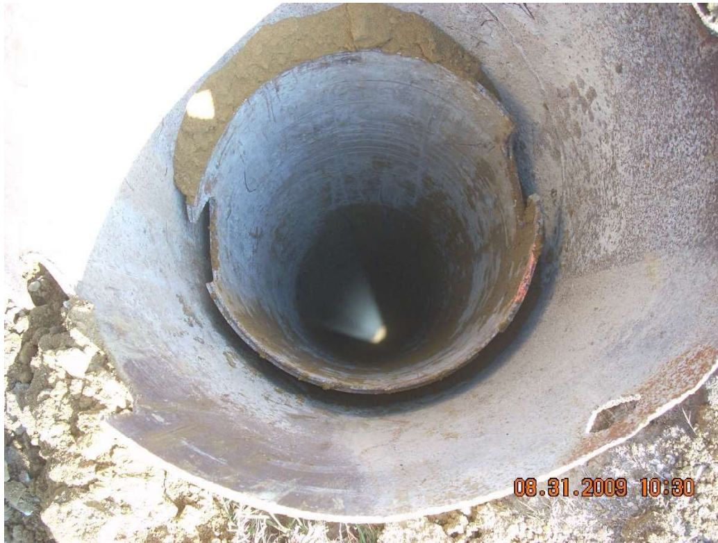
Figure 5-9 Use of Telescoping Casing to Complete a Dry Excavation at a Site Near Dallas, Texas
