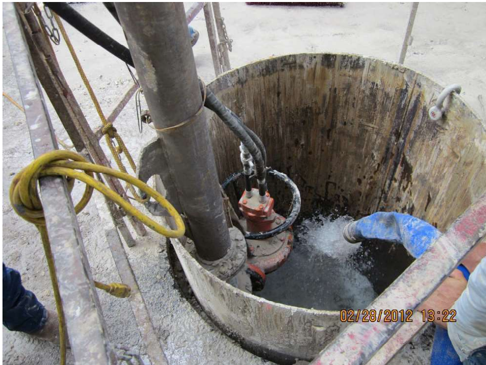
Figure 5-36 Hydraulic Pump for Cleaning Bottom and Pumping Slurry
