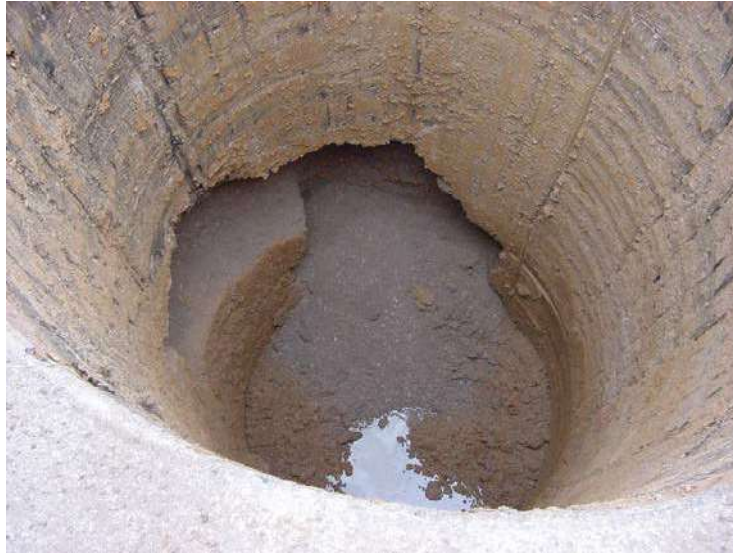
Figure 5-40 Caving in an Unsupported Drilled Shaft Excavation
