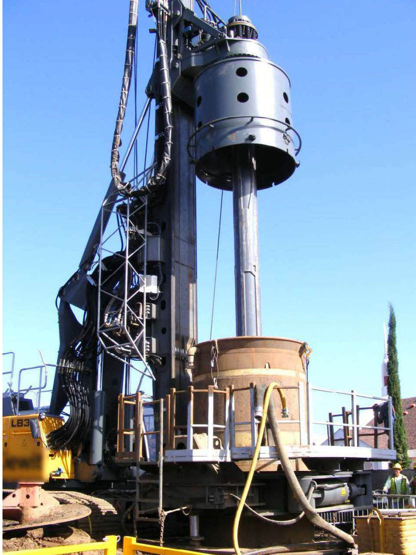
Figure 5-13 Segmental Casing Installed with an Oscillator Attachment to a Hydraulic Drill Rig
