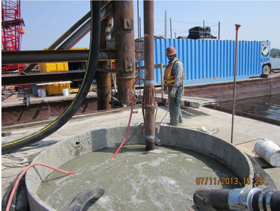
Figure 5-35 Airlift Pump for Cleaning Bottom and Pumping Slurry
