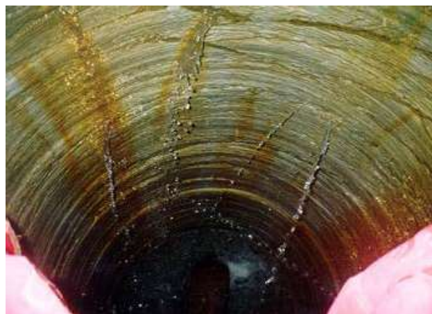
Figure 5-23 Excessive Seepage into a Drilled Shaft Rock Excavation (photo courtesy of PennDOT)
