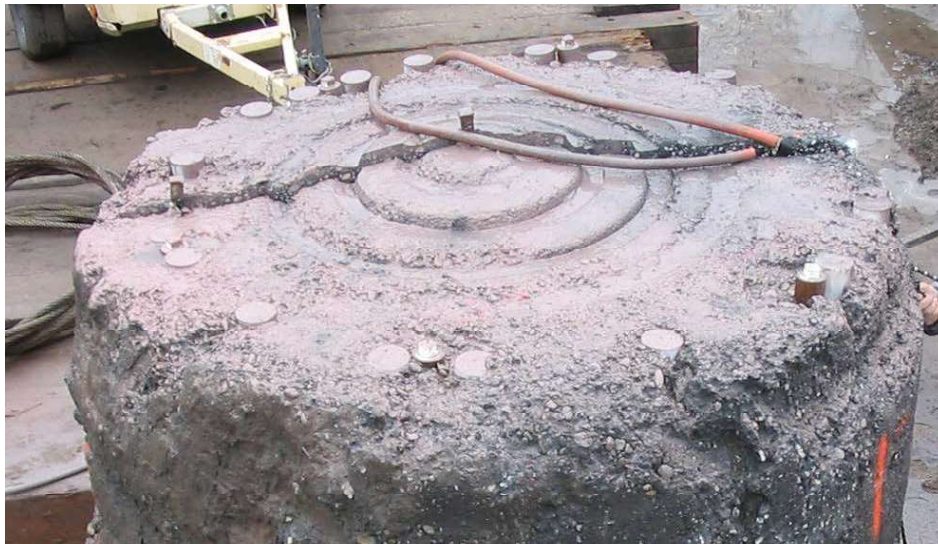
Figure 5-37 Photo of the Base of an Exhumed Drilled Shaft, Cast Under Drilling Fluid
