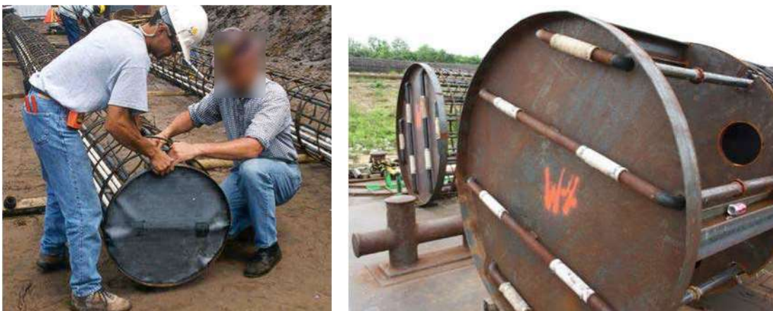
Figure 3-16 Post Grouting Devices Attached to Reinforcing Cage: Flat-jack device (left) and Tube-a-manchette device (right)
